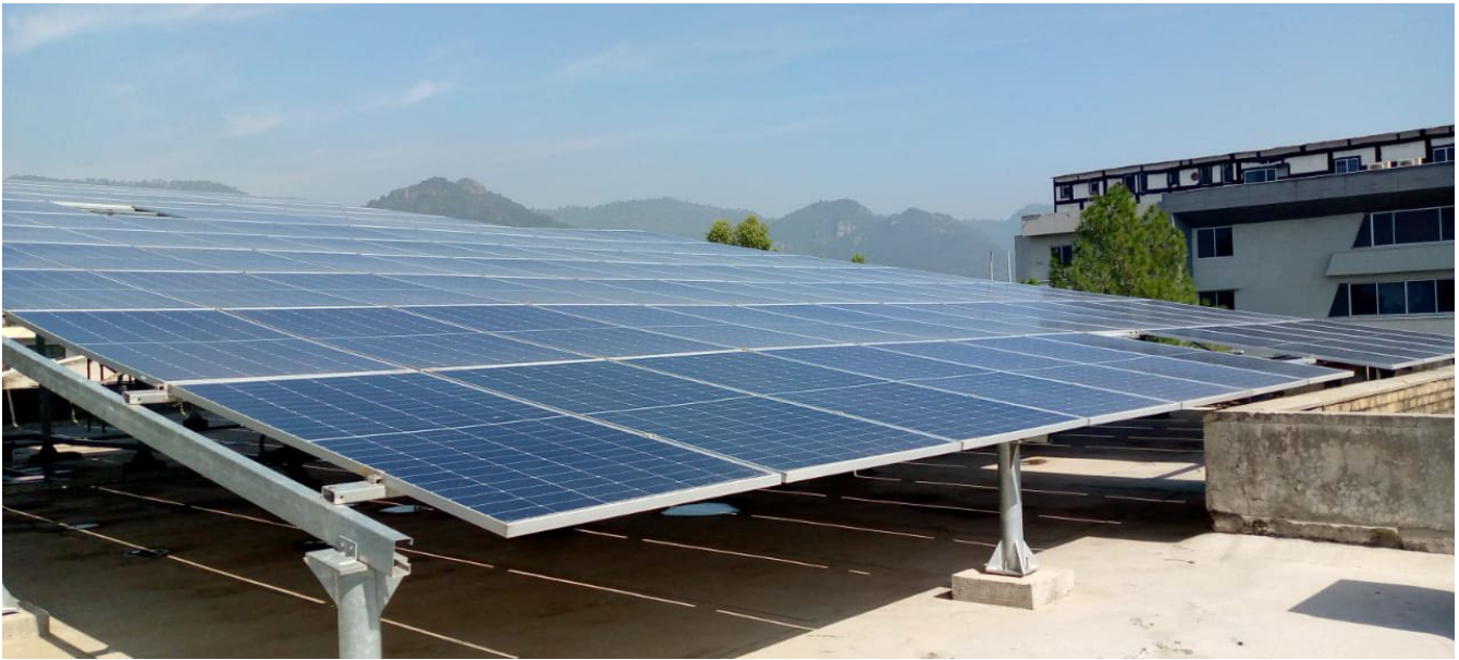
230Kva Solar Energy System
